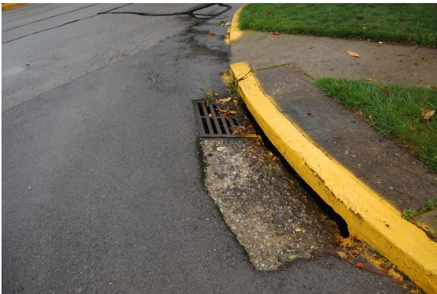
Storm drain in neighborhood. Image Citation: A. Osborne, UK CAFE.
